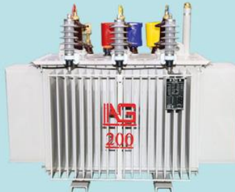
200 kVA, 11/0.4 kV, NLTC -7 Pole Mounted Transformer
