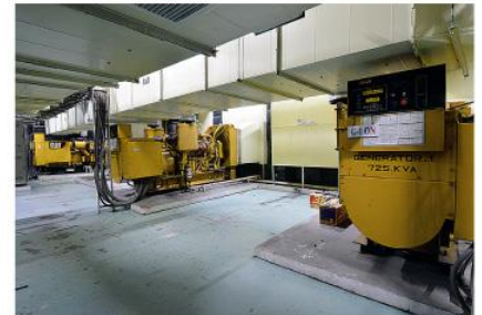
▲ Generally generators are installed on the first floor and underground, but here it was installed on the 4th floor to avoid flooding. That way, a stable power supply is accomplished.
