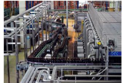
The performance of bottling line which was low at the time has been improved dramatically. PDCA cycle is thoroughly executed.
