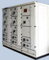
Main Distribution Board
