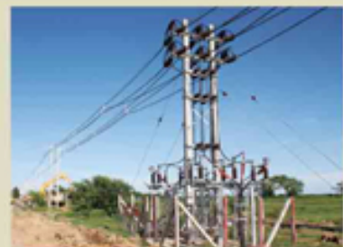
Electricity supply network has been built by using Yen loan.
